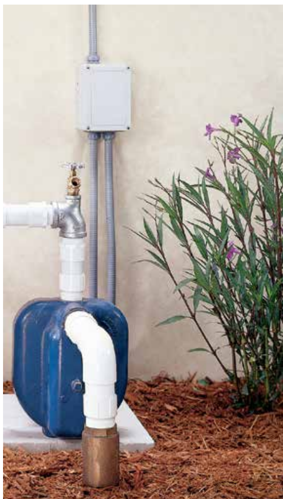
pump start relays
