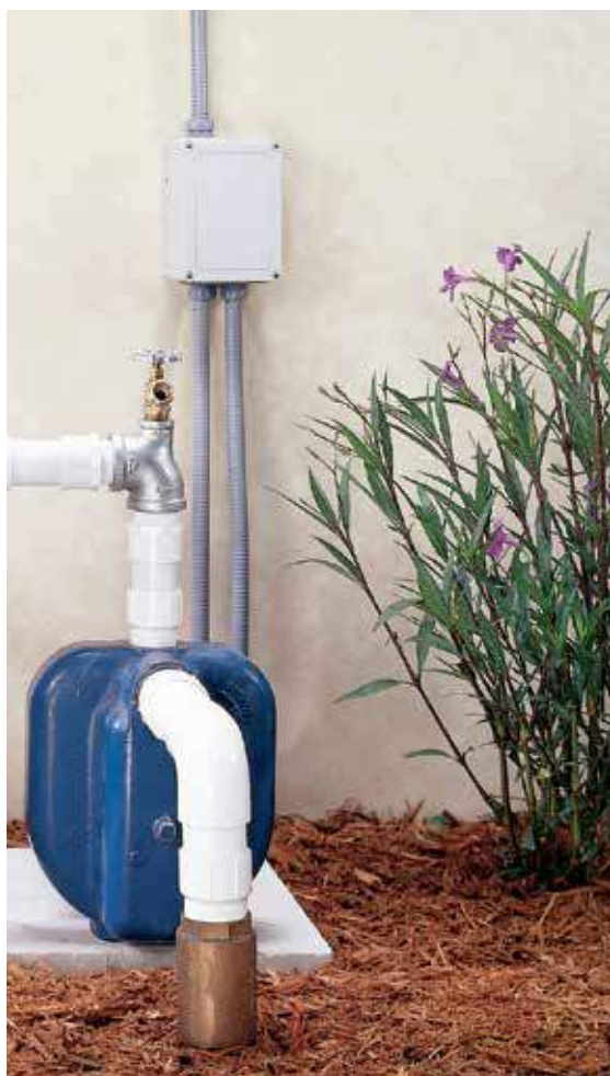
pump start relays
